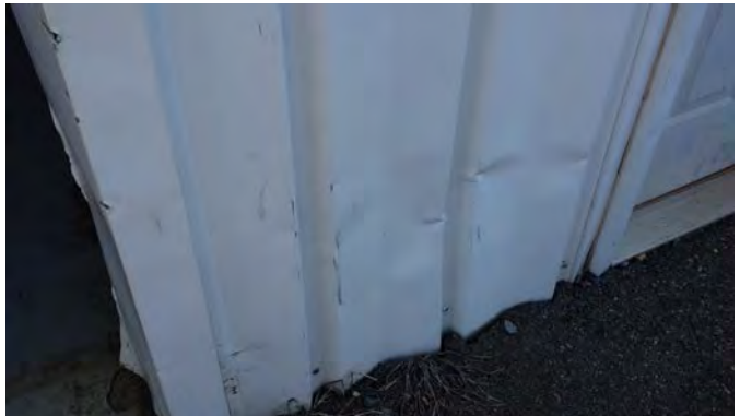
Dented Metal Wall Panels - Few Locations
