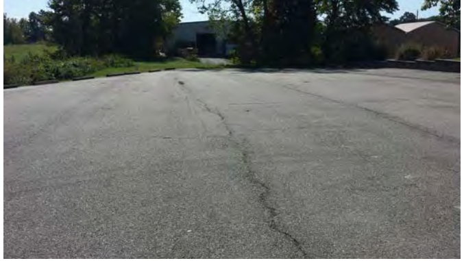
Front Parking Lot - Minor Cracking in Paving
