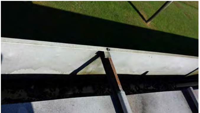
Typical Cutter - Minor Ponding of Water
