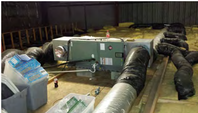
HVAC Unit Above Fitness Center at 1950 Metal Building
