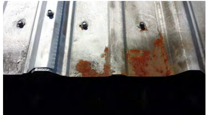
Typical Condition of Screw Down Metal Roof at 1967 Metal Building (Borum Shop)
