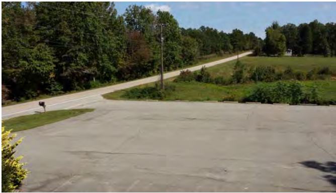
Front Parking Lot - Minor Cracking in Paving
