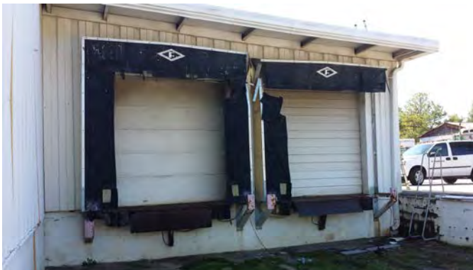
Dock Levelers and Dock Seals at Loading Dock
