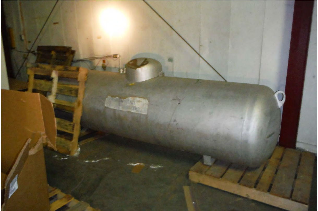
30. Empty propane tank observed in the northern warehouse.
