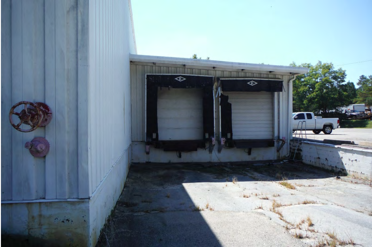
11. Loading docks and stormwater drain (below docks) observed on northern side of building.
