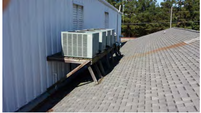
Condensing Units Serving Office Area Fitness Center
