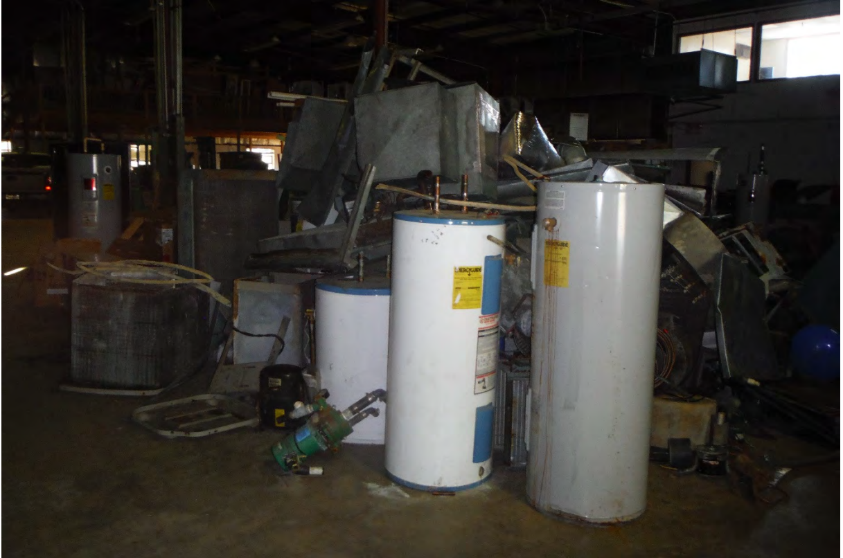
39. Water heaters and AC fan unit observed in southern warehouse.
