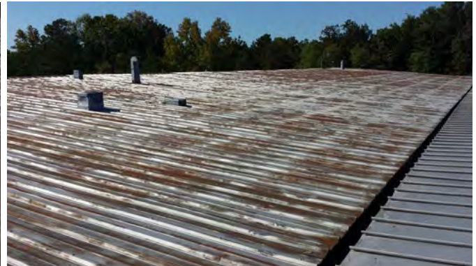
Typical Condition of Screw Down Metal Roof Over 1967 Metal Building (Borum Shop)
