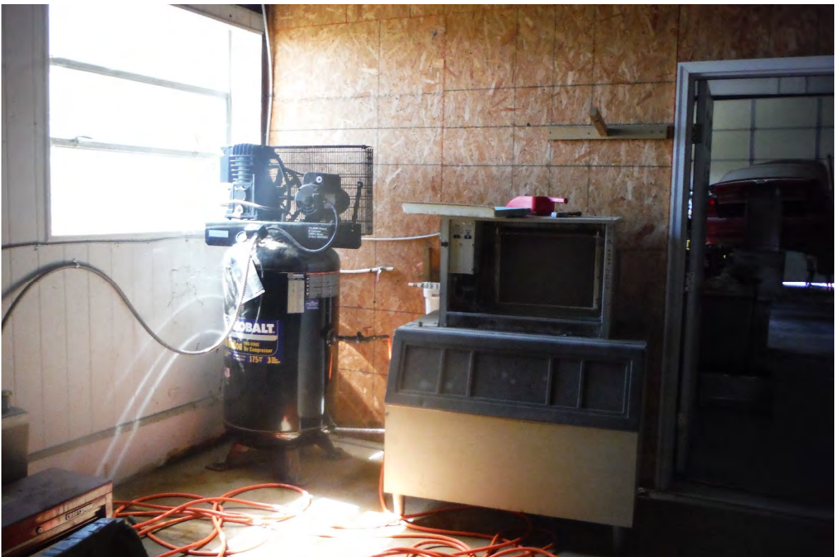
40. Air compressor observed on the southern wall of the warehouse. No staining was observed around the air compressor. The door shown on the right side of the photograph leads to a metal working and car lift room located at the southwestern corner of the building.
