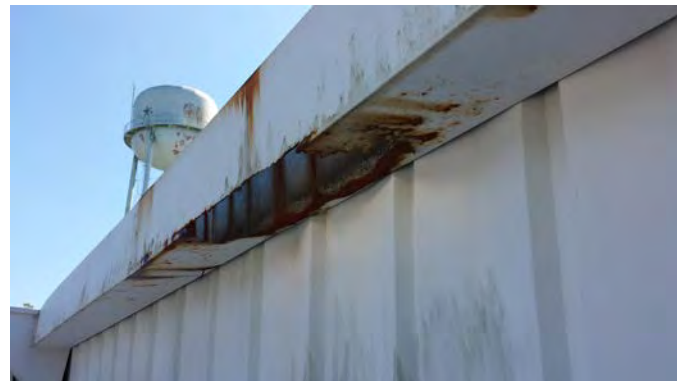
Rusted Gutter on Higher Roof (2 locations) Adjacent to Loading Dock Roof
