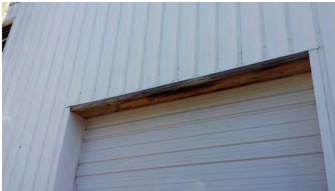
Aluminum Trim Missing at 1967 Metal Building (Borum Shop)
