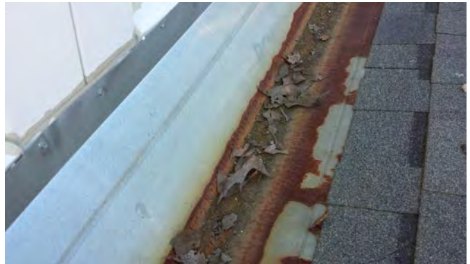
Roof to Wall Flashing at Shingle Roof to Metal Building Wall Panels
